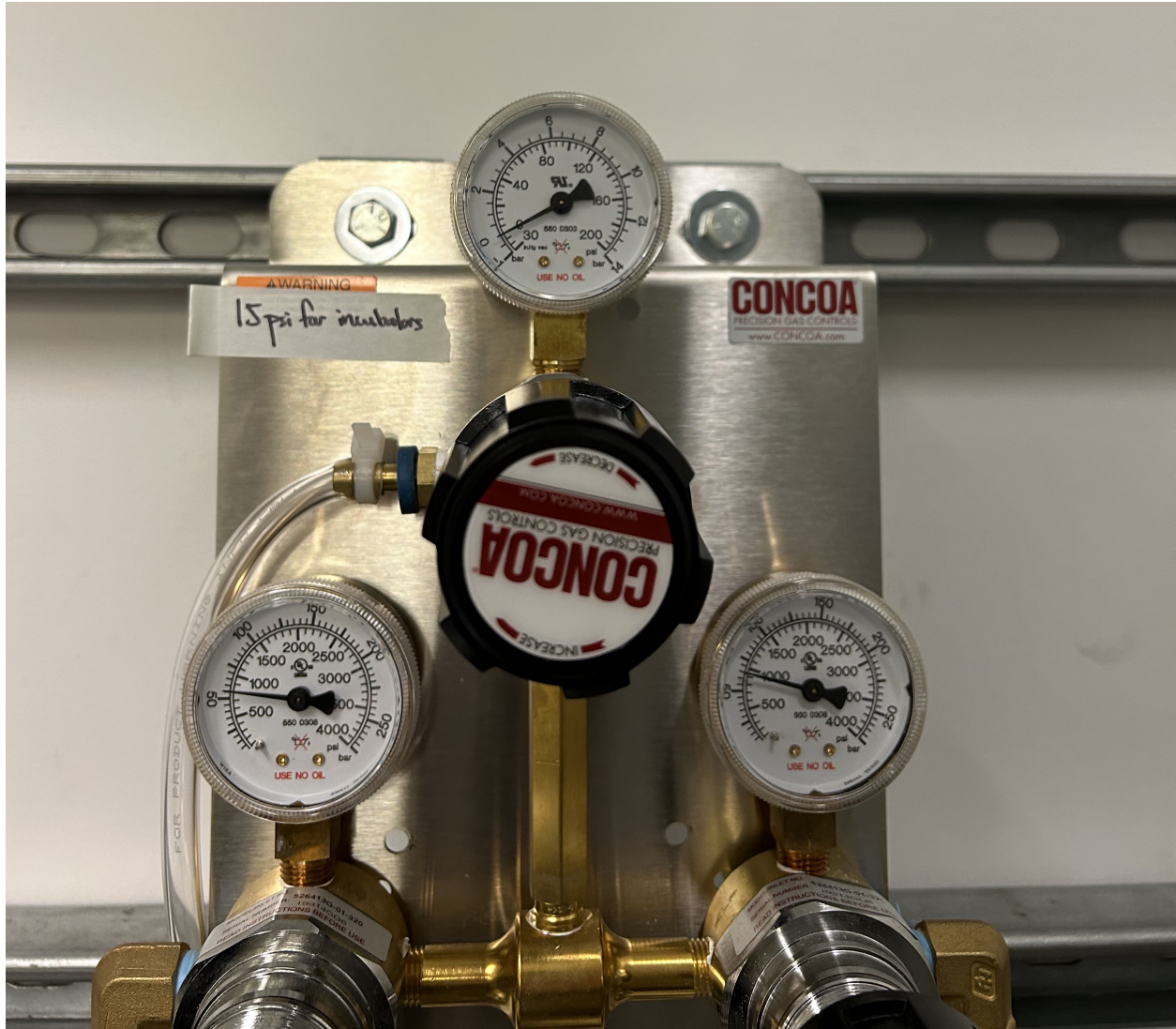
Fig. 5: Carbon dioxide knob (black, center) and pressure gauge (top, currently at 0 psi).
